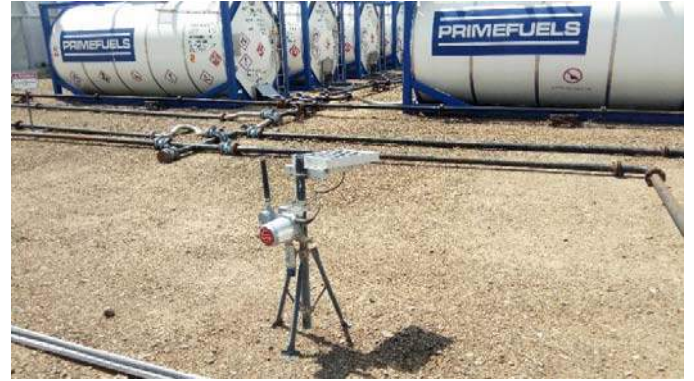
2. Gas detection within 15 meters of loading area
